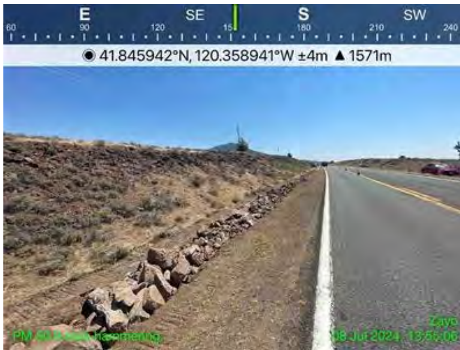
Figure 1. View to south of rock hammer working along fiber trench in the Northern Area (Modoc County).
