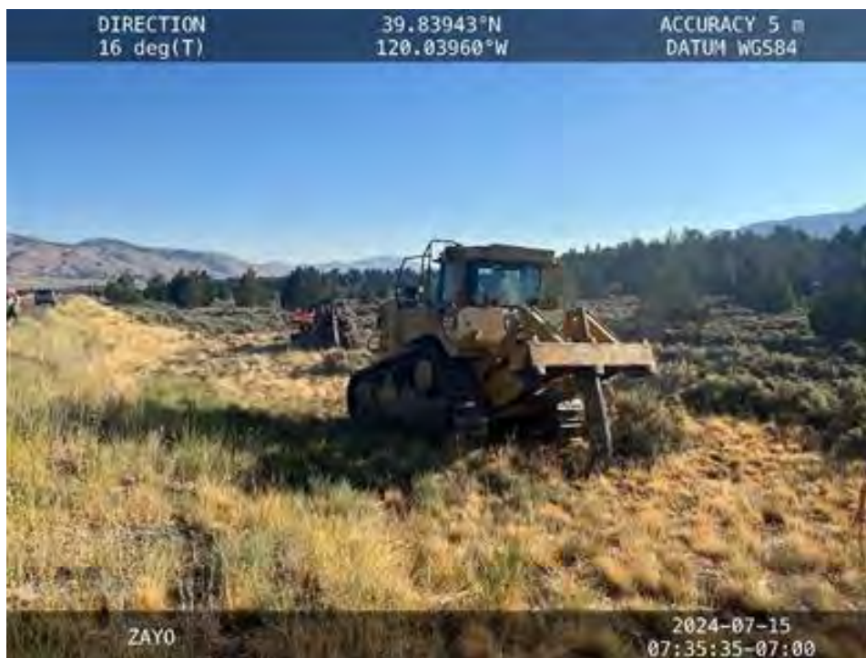
Figure 4. View to the north of pre-ripping operations in the Southern Area (Lassen County).
