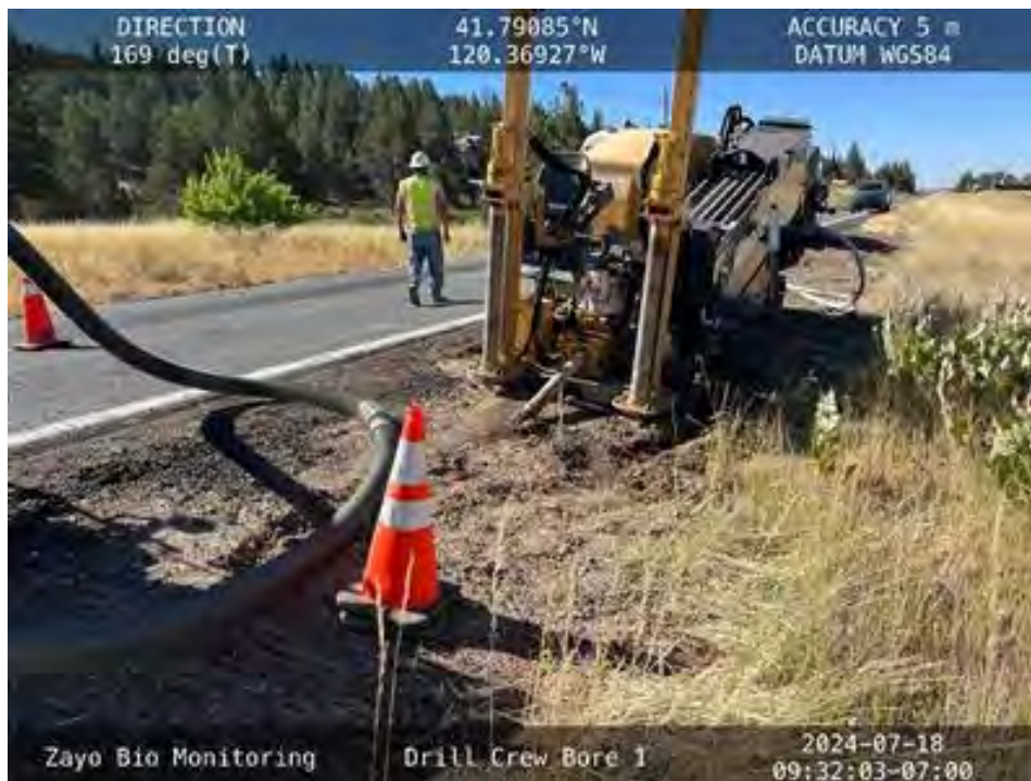
Figure 8. View to the south of HDD shot in the Northern Area, Modoc County.
