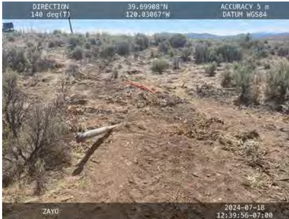
Figure 7. View to the southeast of HDD shot that has been completed (Southern Area, Lassen County).
